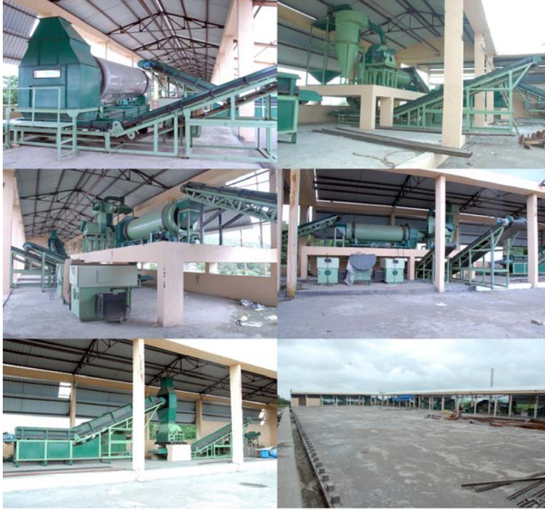
RDF PROCESSING UNIT
