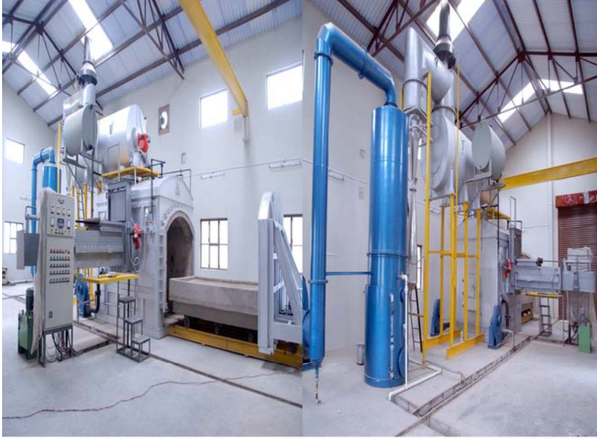
DEAD ANIMAL INCINERATOR
